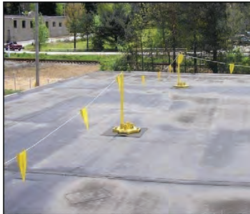
Warning Line System
