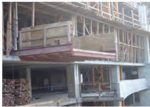
Loading Platform w/Removable Chain at point of access, however Mid Rail is also Required
