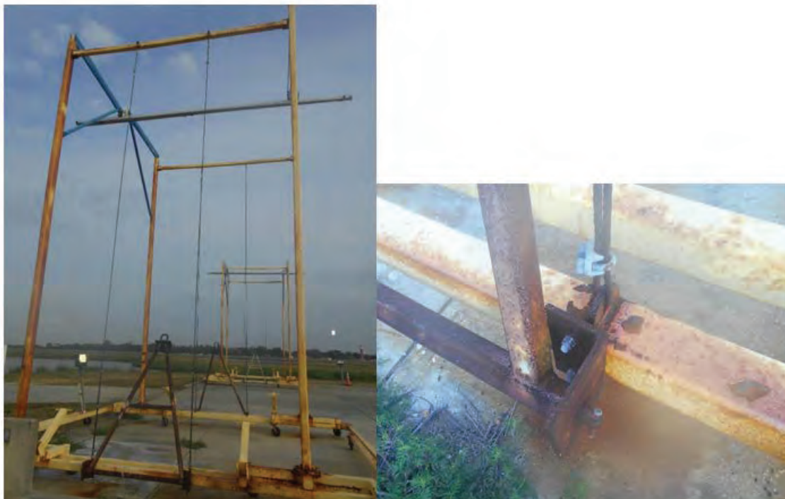
Figure 5. Corrosion issues noted on Webb-Rite Overhead Rigid Rail Systems located at the wash rack.
