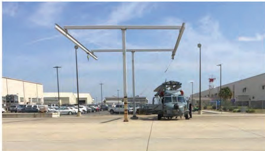
Figure 12. Wash rack facility.
