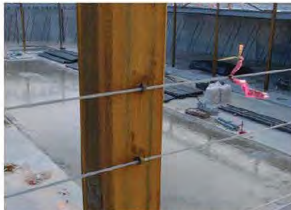
Steel Cable Guardrail
