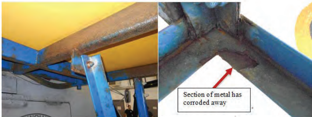
Figure 3. Corrosion issues noted on Blue Webb-Rite work stands.
